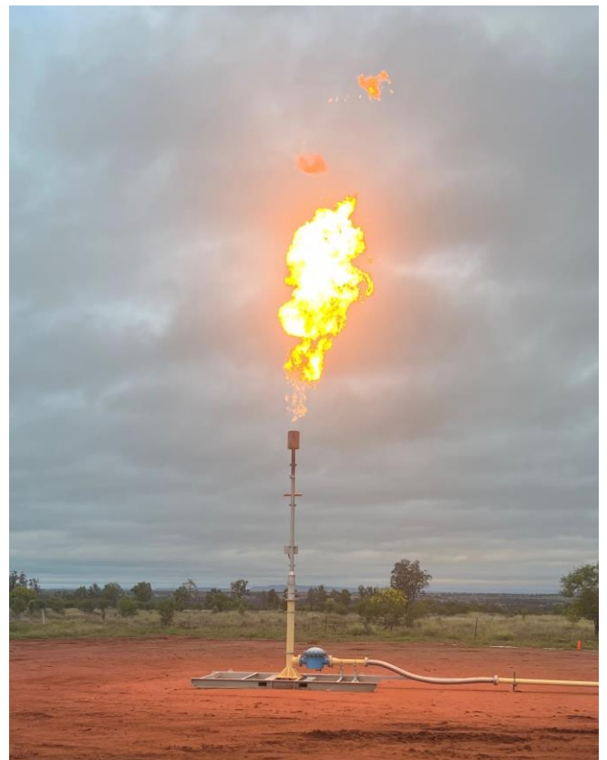
Figure 3 – Mahalo North 1 flare
